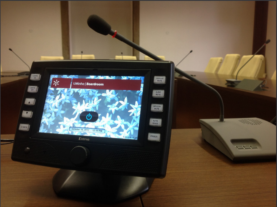
UMINHO COMPLETE MEETING ROOM SOLUTIONS CONTROL & AUTOMATION
